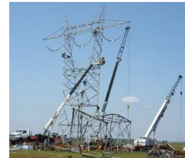
TVA rebuilt towers and ran a dedicated line to restore our power source.
